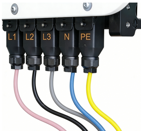
Figure 7- 19 Backup port auxiliary cable connection
